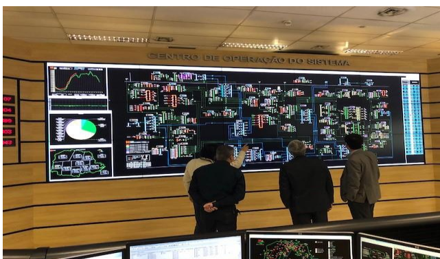
USTDA visit to Brazilian utility Copel's central control room
